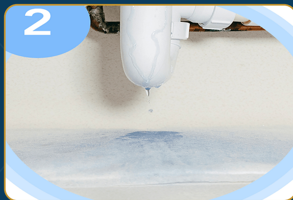
Catching drips at the trap
